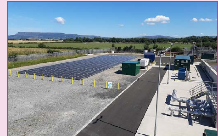
Solar powered battery energy system at Ballykelly wastewater treatment works, County Derry/Londonderry.
