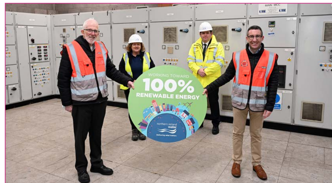
Piloting the production of green hydrogen - NI Water staff showing Alliance Party of Northern Ireland MLA's Andrew Muir MLA and Stewart Dickson MLA the 10kW Electrolyser at Kinnegar Wastewater Treatment Works in Belfast.
