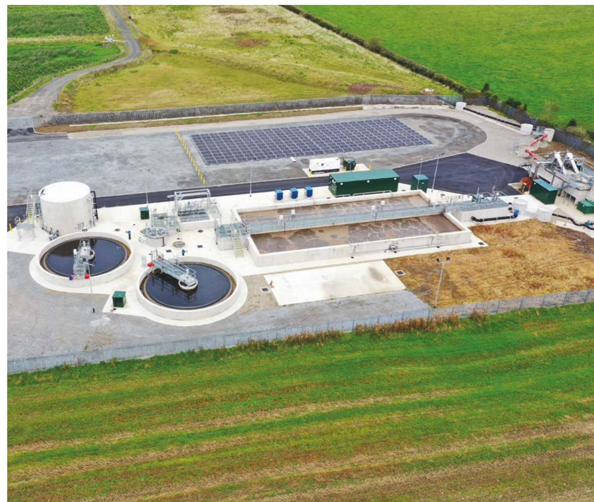
Battery and solar panel system at Ballykelly wastewater treatment works, County Derry/Londonderry.
