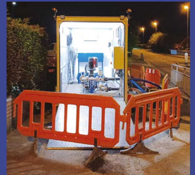
NI Water's new custom-made pumping trailer.
