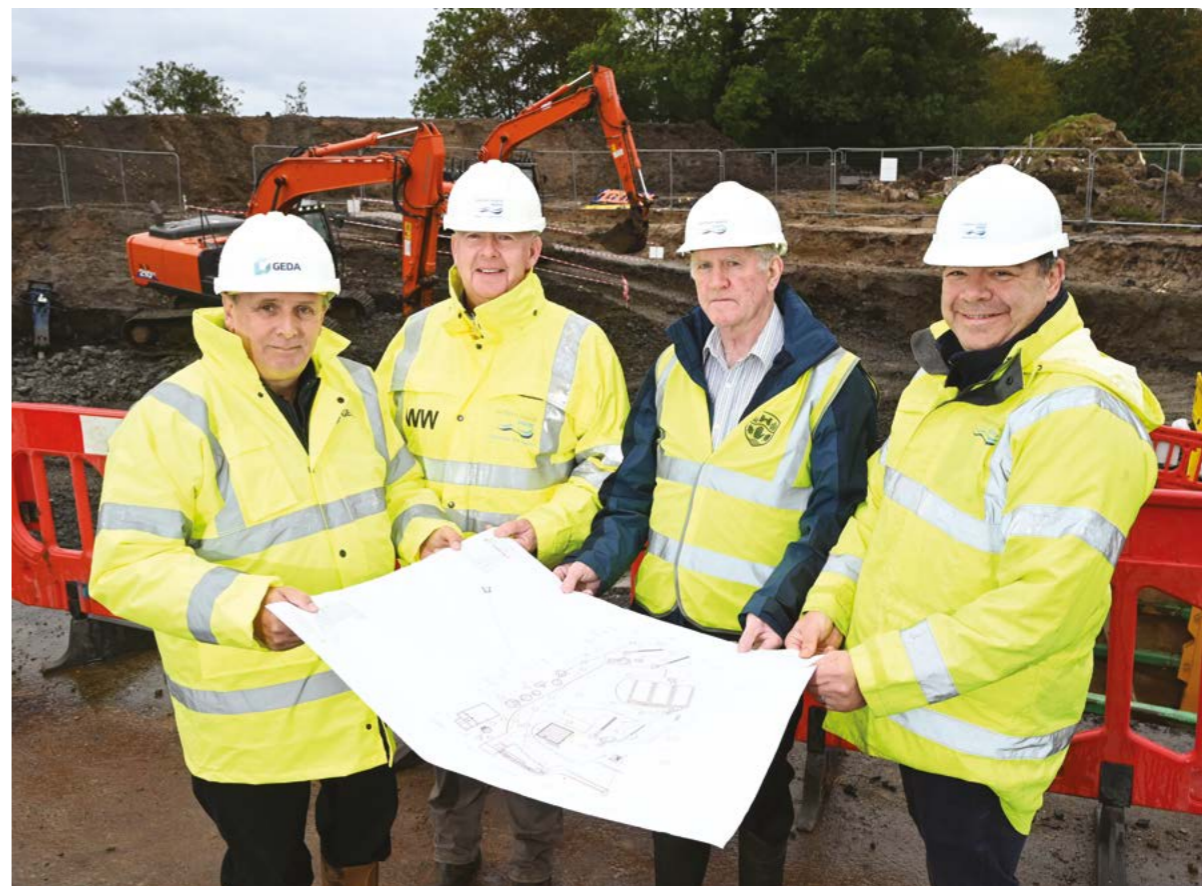
NI Water break ground on the new £4.8m Ballyronan wastewater treatment works, County Derry/Londonderry.
