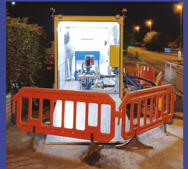
NI Water's new custom-made pumping trailer.
