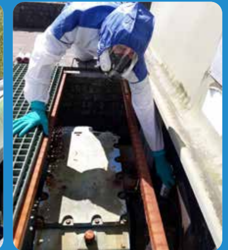
Mechanical and electrical operative fitting a greaser
