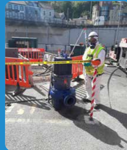
Submersible pump removal from 11 metre wet well at a wastewater pumping station
