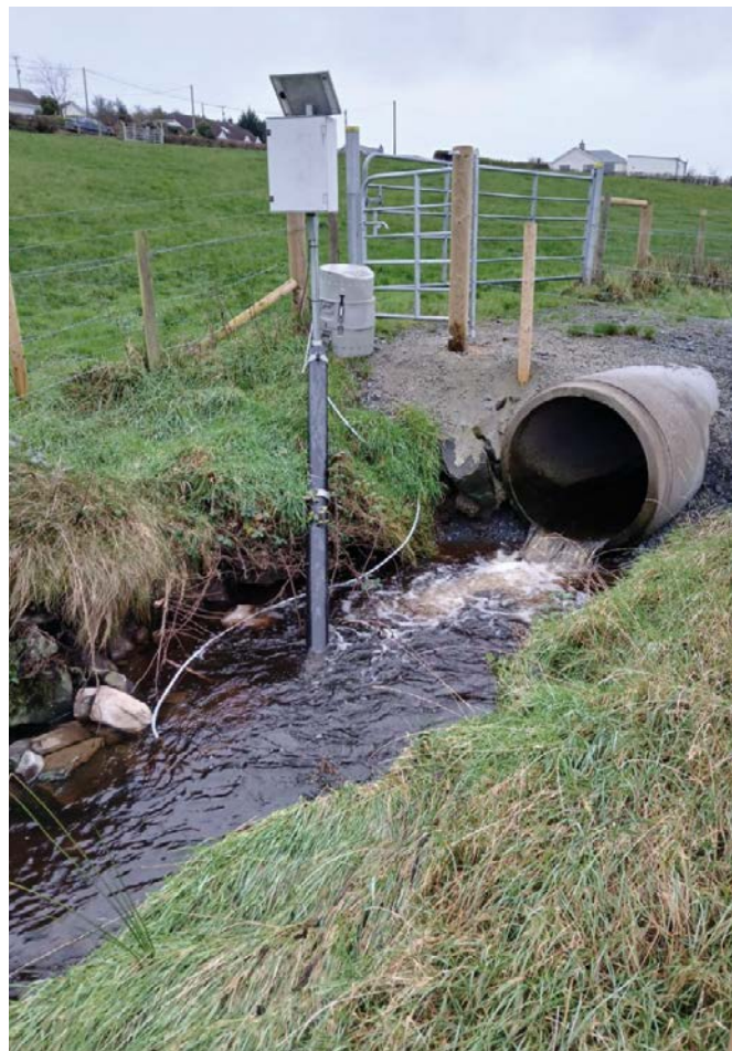
Figs 6 and 7: Water quality monitoring equipment installed in the clay Lake catchment, with solar power units
