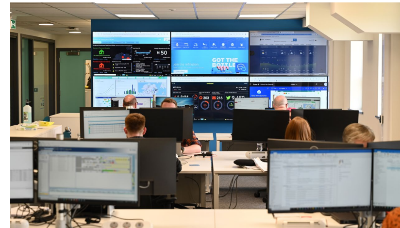
NI Water's Intelligent Operations Centre.
