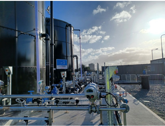
Hydrogen and Oxygen Demonstrator Project at Belfast wastewater treatment works, County Antrim.
