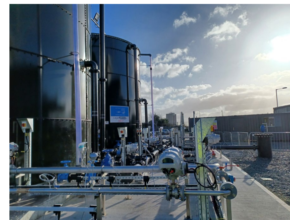
Hydrogen and Oxygen Demonstrator Project at Belfast wastewater treatment works, County Antrim.
