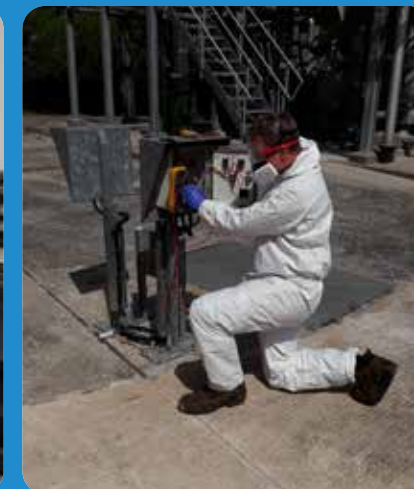
Mechanical and electrical operative checking return liquor pumps
