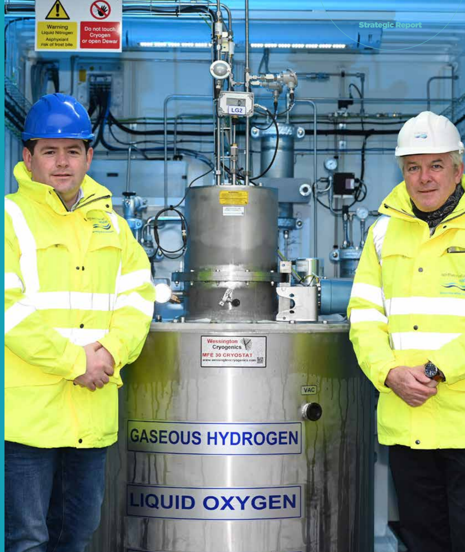
Electrolyser at Kinnegar wastewater treatment works, Hollywood, County Down
