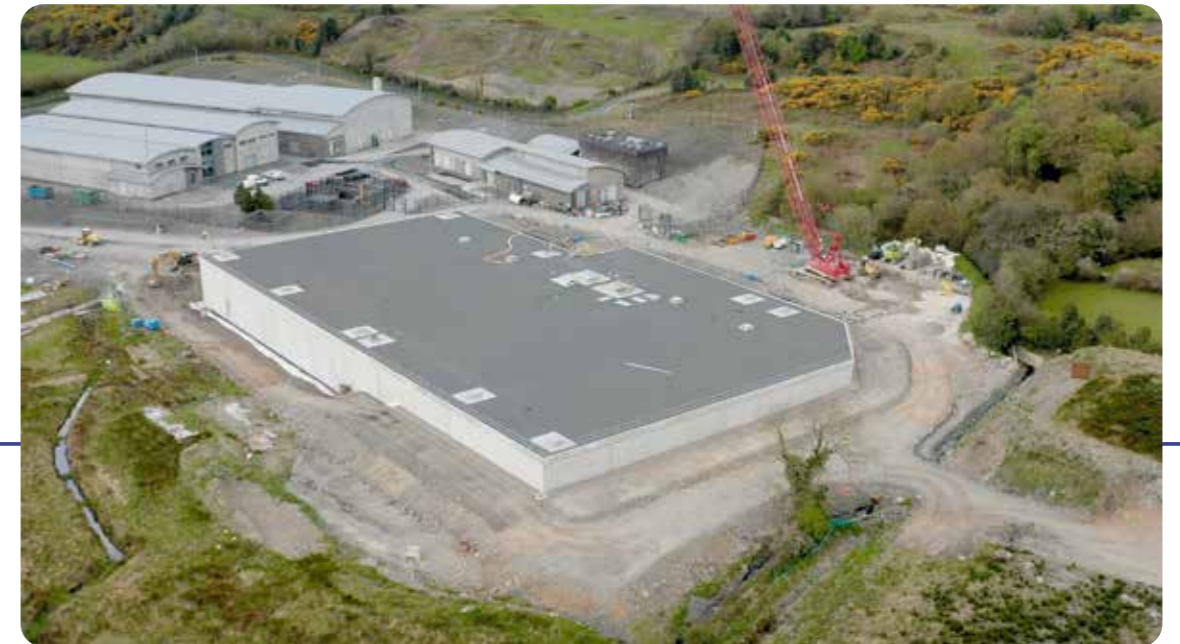
New water storage tank under construction at Drumaroad water treatment works, Castlewellan, County Down
