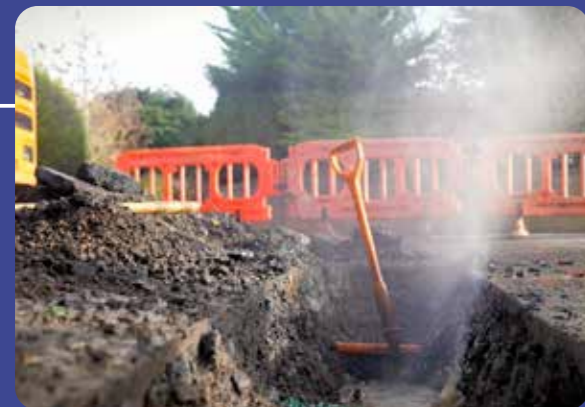
Water leaking from a burst pipe
