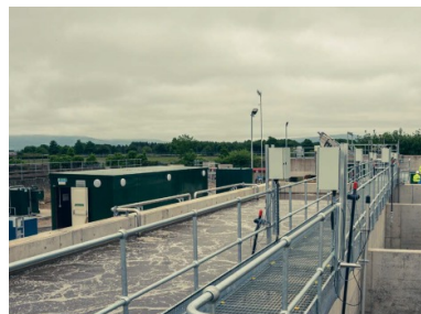
Ballykelly Activated Sludge Process
