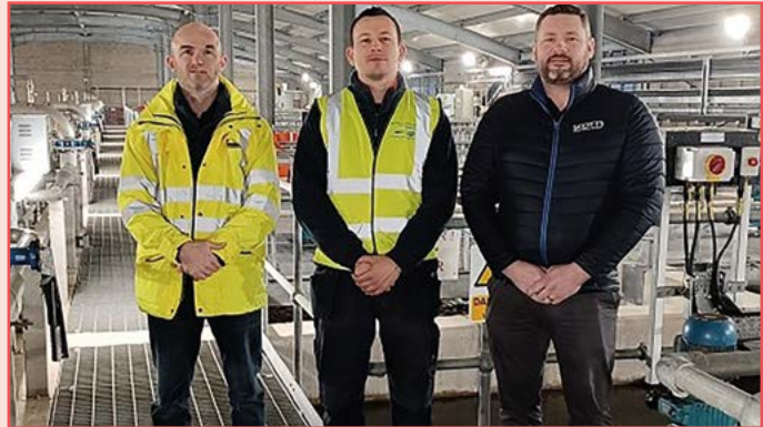
Energy efficiency LED lighting at Drumaroad water treatment works, County Down.
