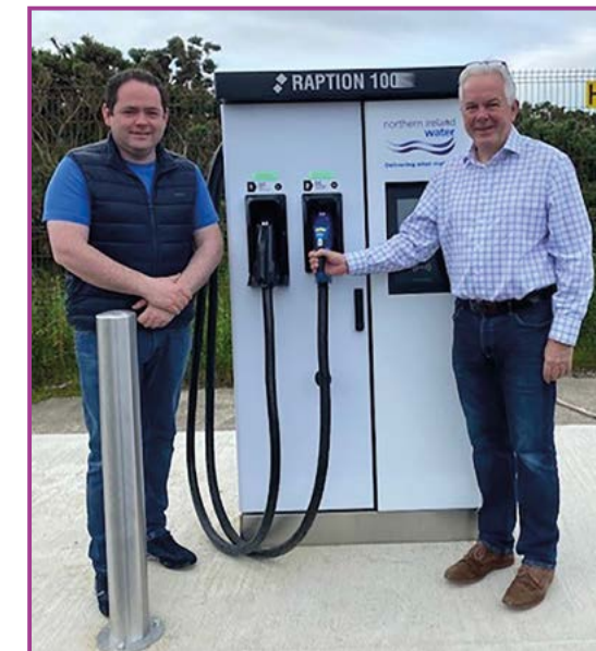
Electric charging infrastructure at one of NI Water's sites.
