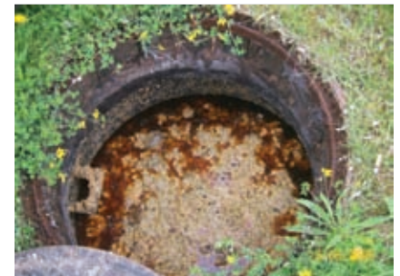
Fat building up in a manhole
