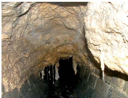
Fat beginning to block a sewer
