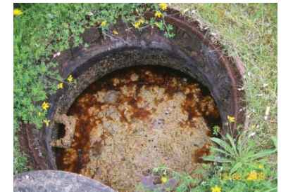
Fat building up in a manhole
