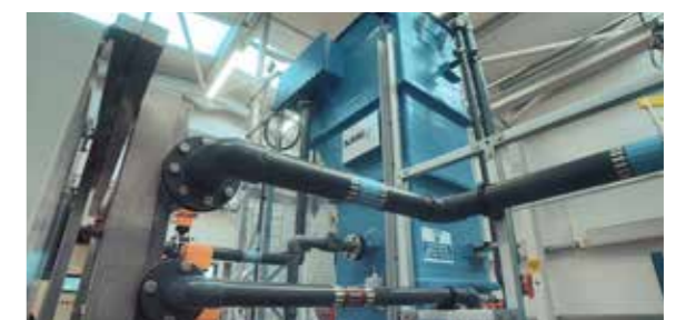
New treatment plant at Rathlin Island, off the coast of County Antrim
